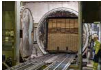
Reactor in Arnhem plant
