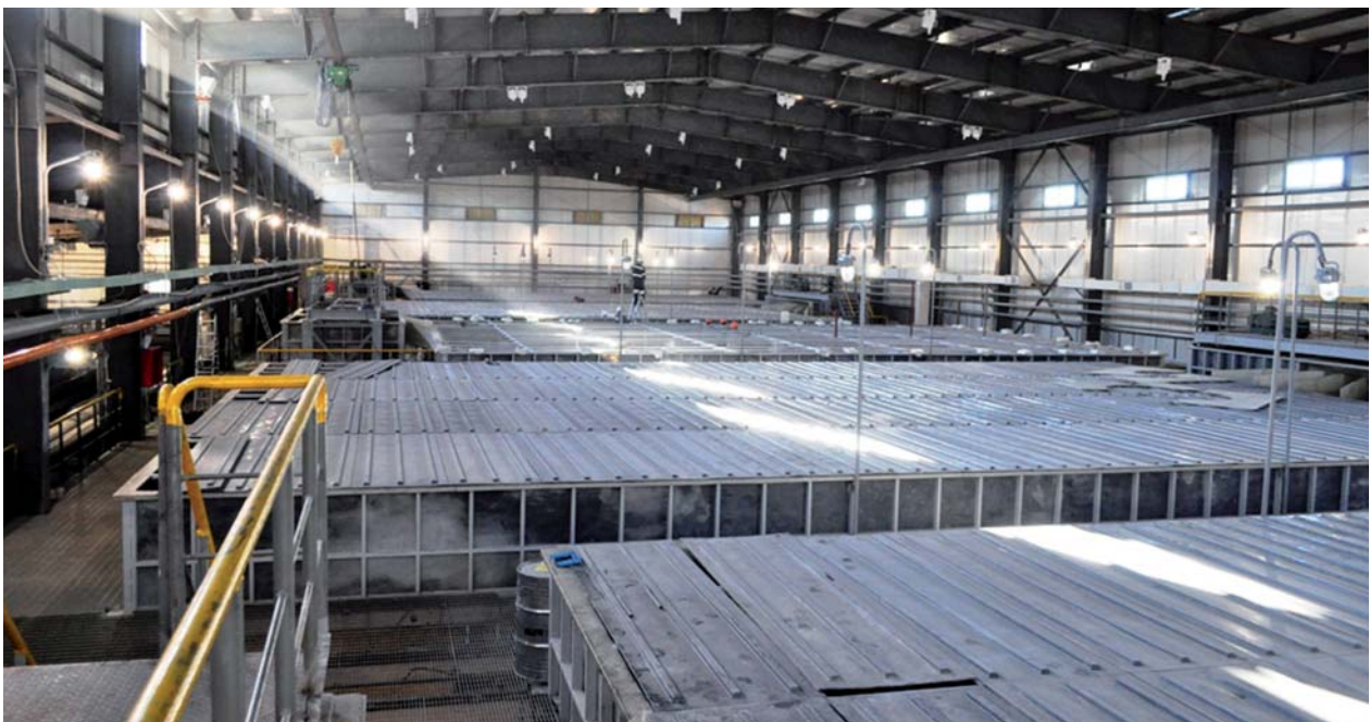
Mixer/Settler tanks – SX plant Kounrad
