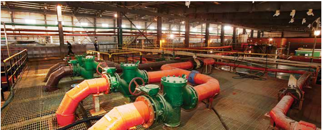
SX building – Kounrad
