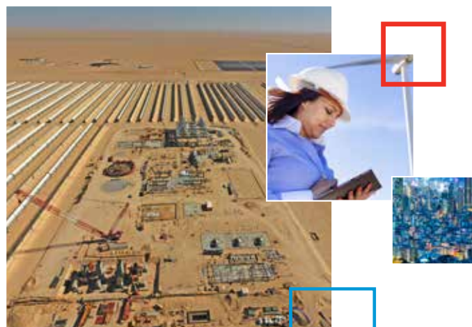
Shagaya Renewable Energy Park, Kuwait. Owner's Engineer and Project Manager, Advisian Madrid. Construction PMC WorleyParsons Kuwait.
