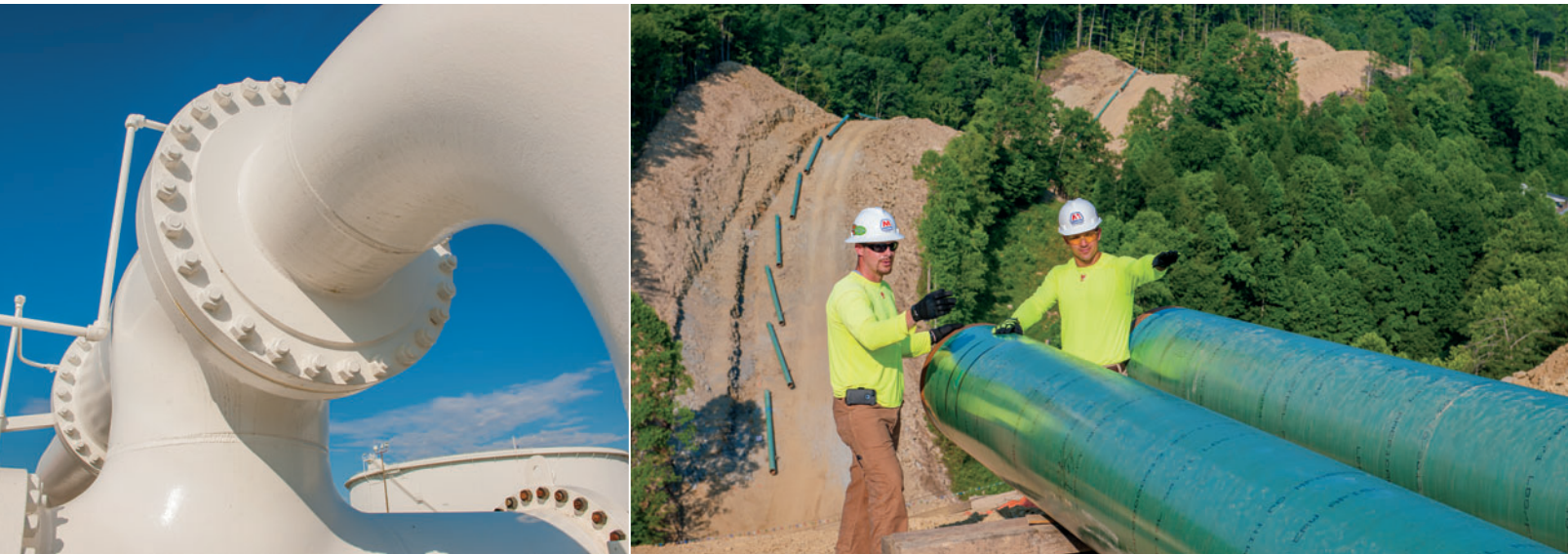
Above: Pipeline at the MPLX terminal in Patoka, Ill. Right: Pipeline construction in Sterling, Ky.
