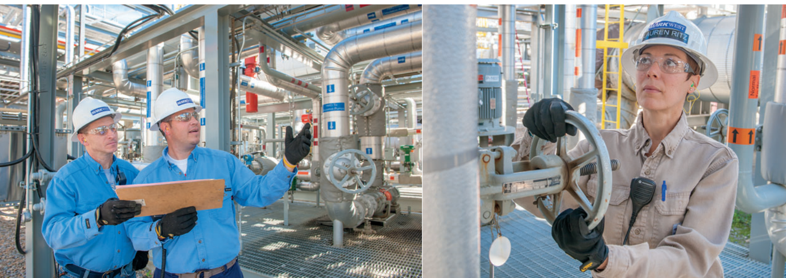
Above and center: MarkWest facilities in Hopedale, Ohio.
