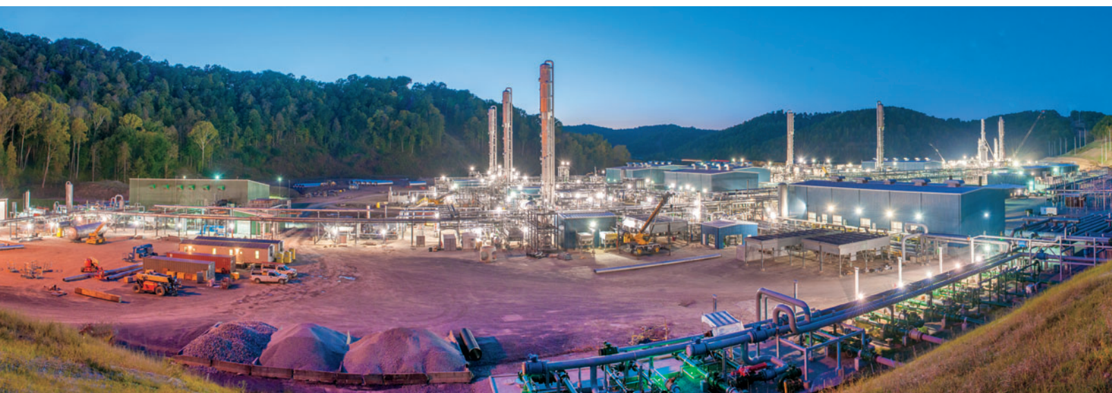
Gas processing facilities of MarkWest's Sherwood complex in West Virginia
