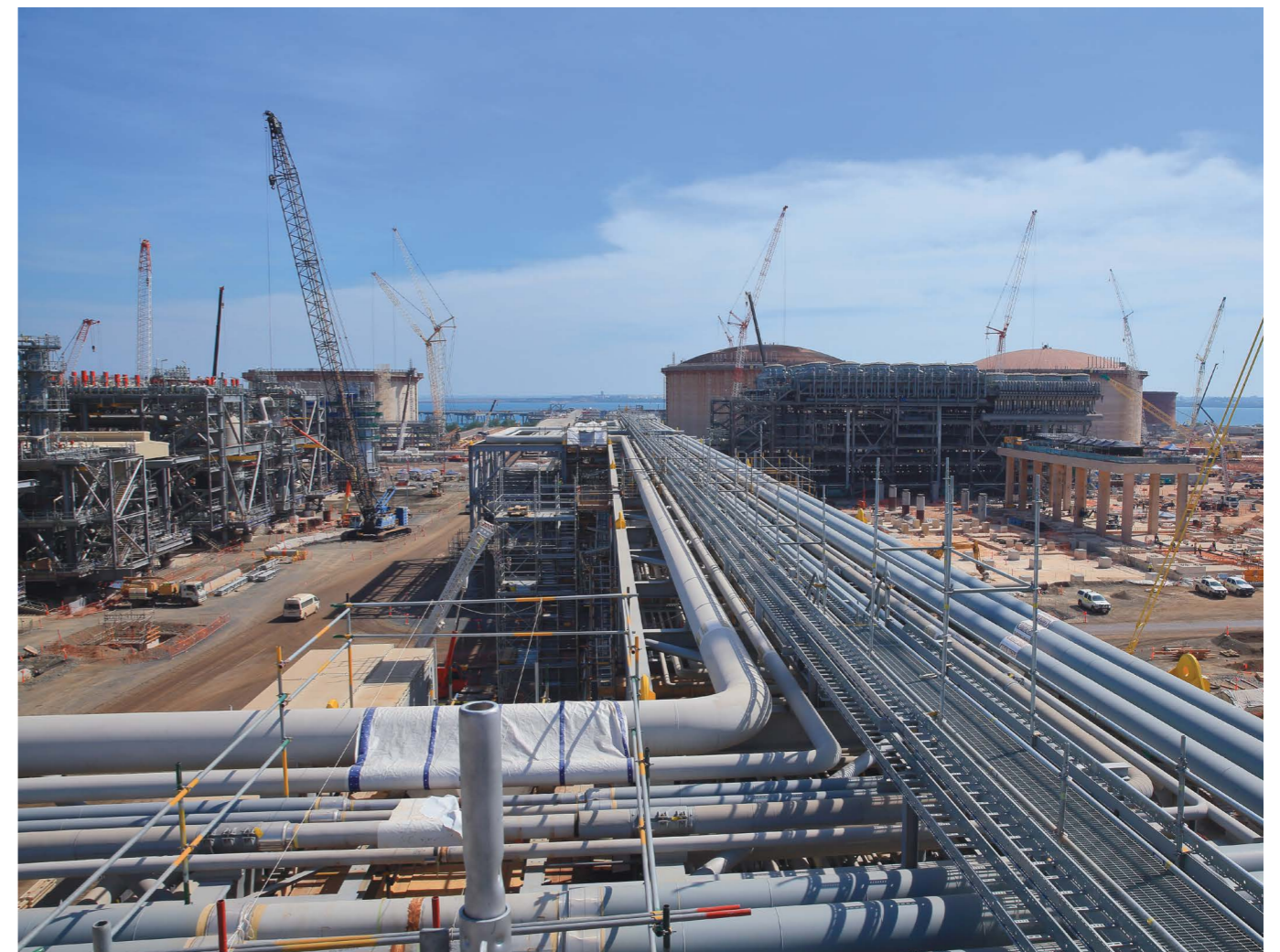
Top Overlooking by-pass module and slug catcher vessel at Spring Gully Pipeline Compression Facility, Roma, Queensland (photo courtesy of Australia Pacific LNG)
