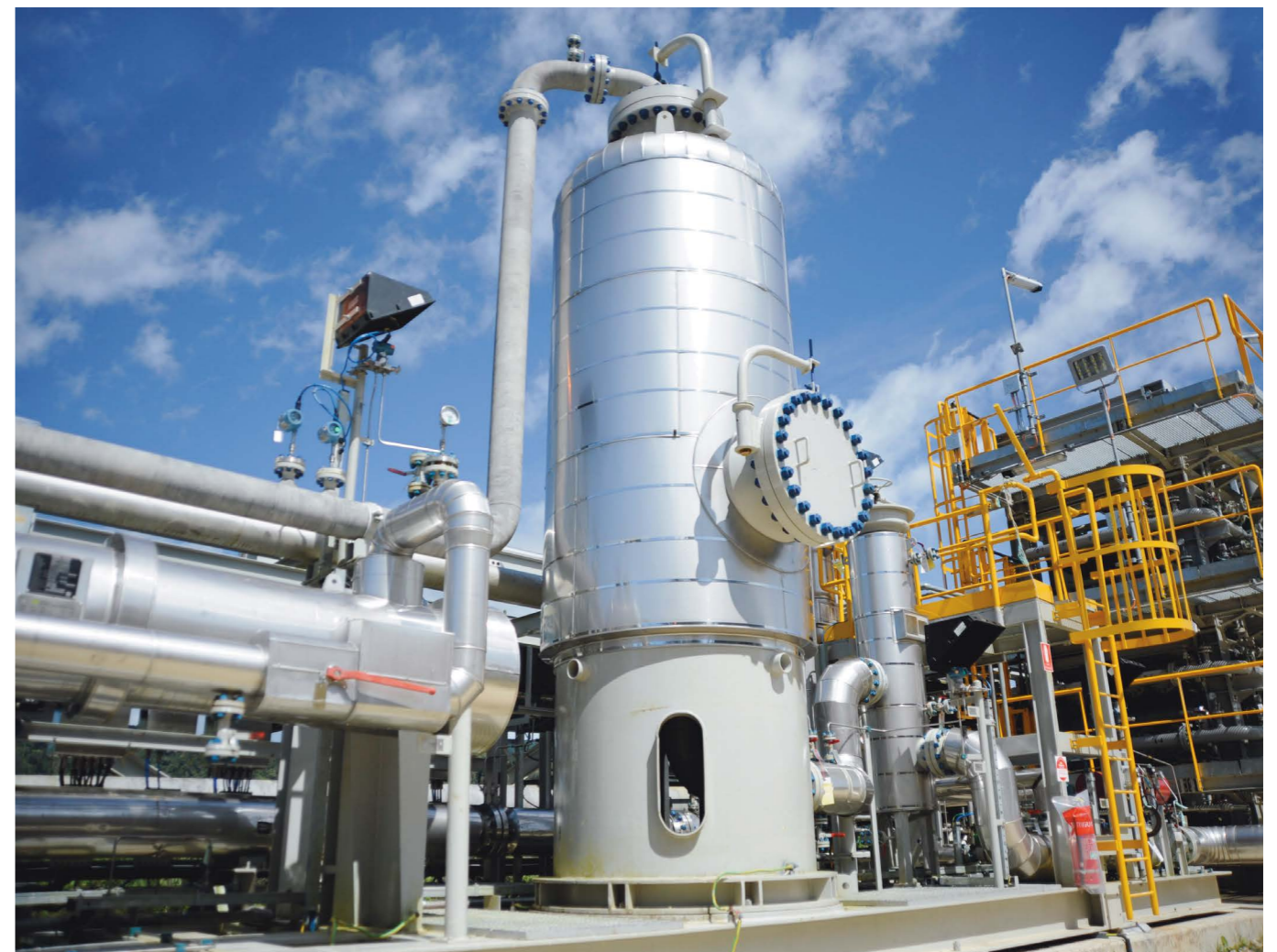
Top Resource Estimator Aaron Brown working at the Dehydration Bed at Karratha Gas Plant, Karratha, Western Australia
