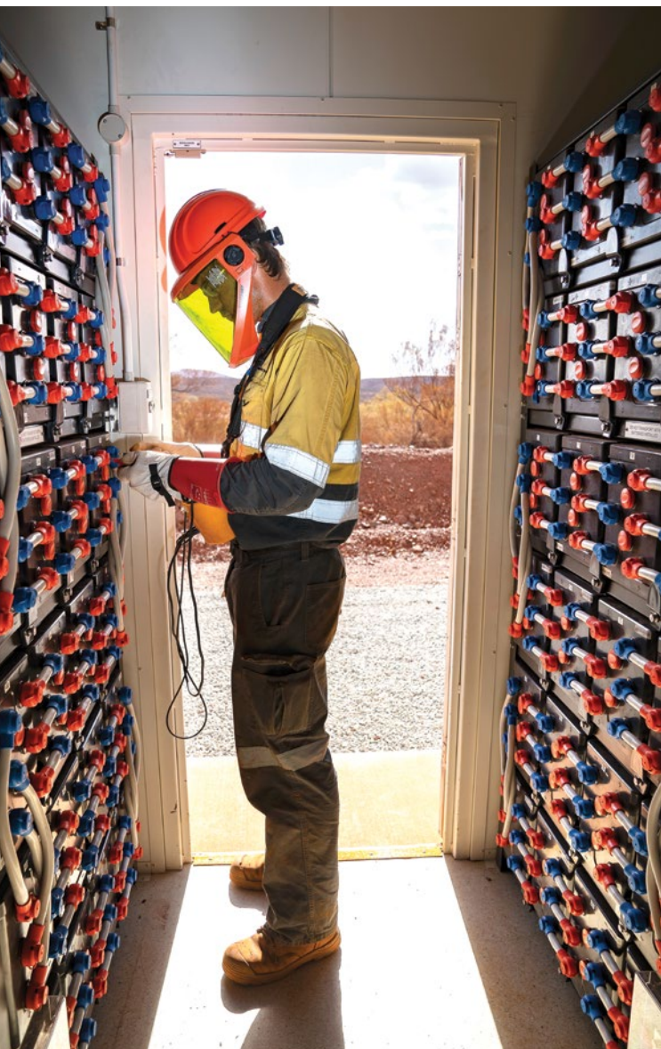
Monadelphous employee testing battery connections during an electrical inspection at BHP's Jimblebar mine, Western Australia.
