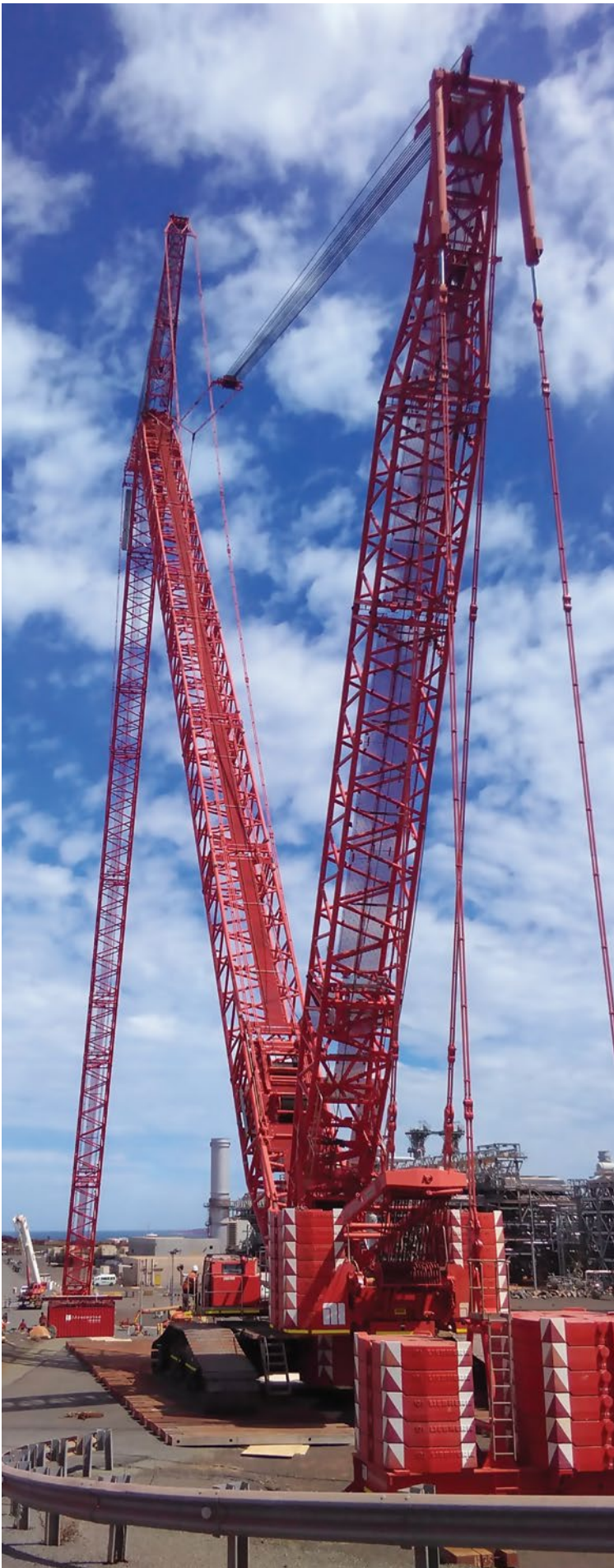
Monadelphous 600 tonne crawler crane preparing to undertake a turnaround at the Woodside-operated Pluto LNG Facility.
