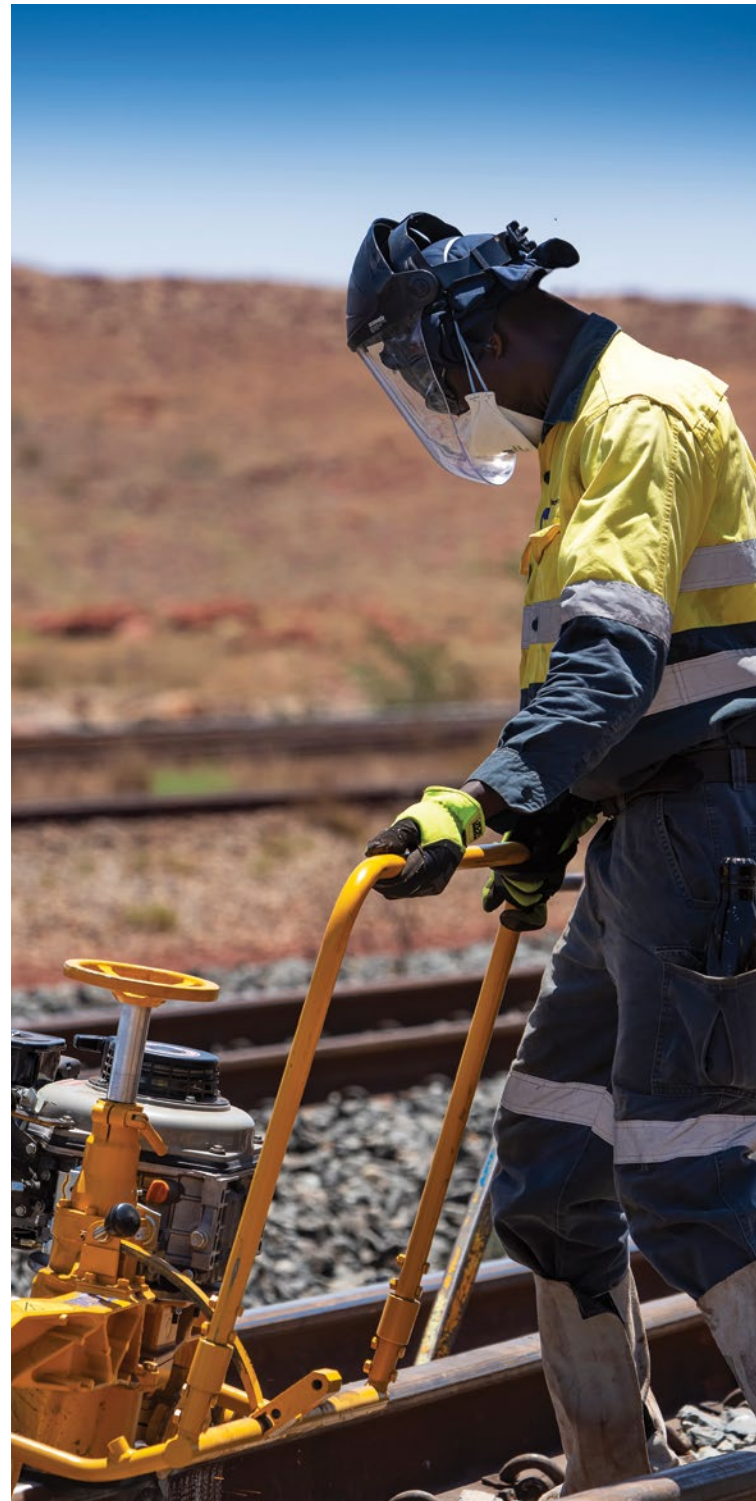
Monadelphous employee using a rail grinder to smooth out an on-track weld outside Karratha, Western Australia.
