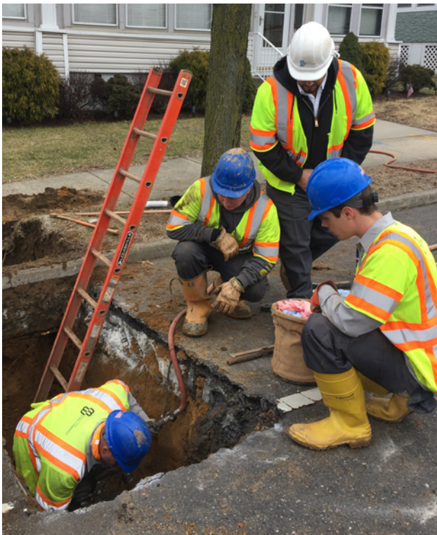
Crew members receive operational instruction and safety training while observing a water main valve replacement.
