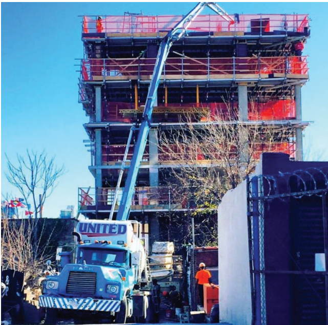
Figure 14. United Transit concrete being supplied to a construction project in New York.
