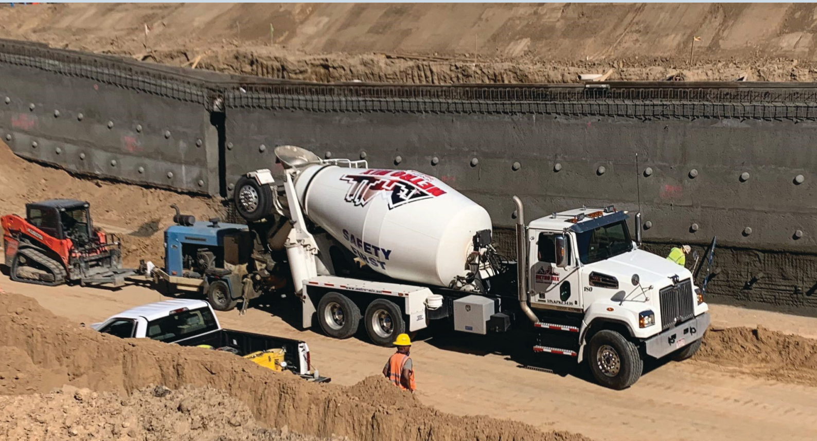
Construction of EdenCrete® enriched concrete retaining walls on Central 70 project in Denver, Colorado
