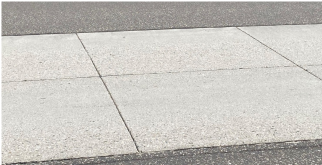
Figure 6 Mid-Section- EdenCrete® Slab – 12 months
