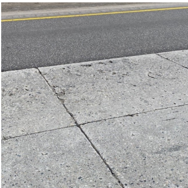
Figure 4 Mid-Section- Reference Slab - 12 months Severe Surface Damage, Joint Rot, Pitting, Pop Outs
