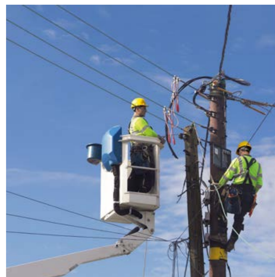
→ Work at height and electrical work related to roll out of networks requires us to insist on strict health & safety requirements for all those working on behalf of Nokia.
