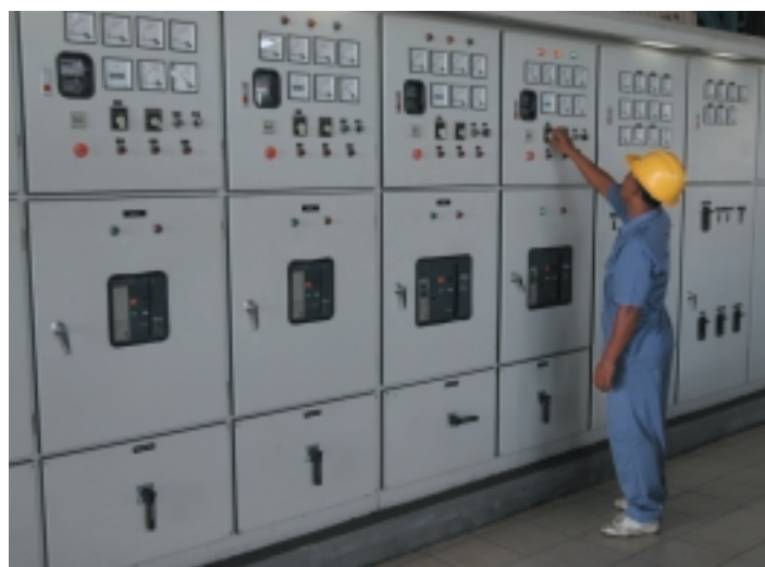
The control room in Pangkatan palm-oil mill.
