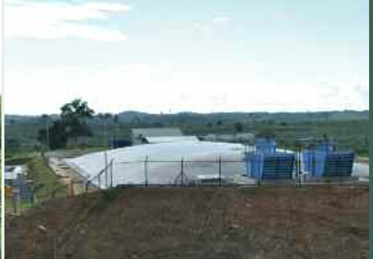
The new electricity-generating biogas plant in Kalimantan
