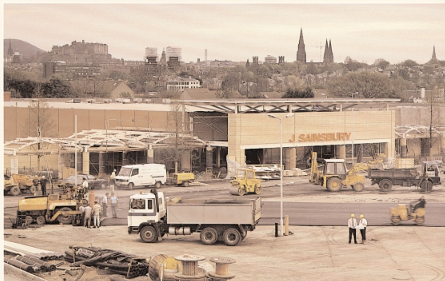
Our Edinburgh store at Blackhall under construction, due to open in June. This is our second supermarket in Scotland and is part of our programme to expand into new trading areas.
