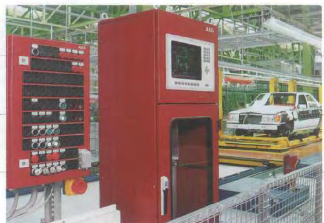
Decentralised operating and viewing station for materials handling equipment at the Mercedes-Benz Rastatt plant.
