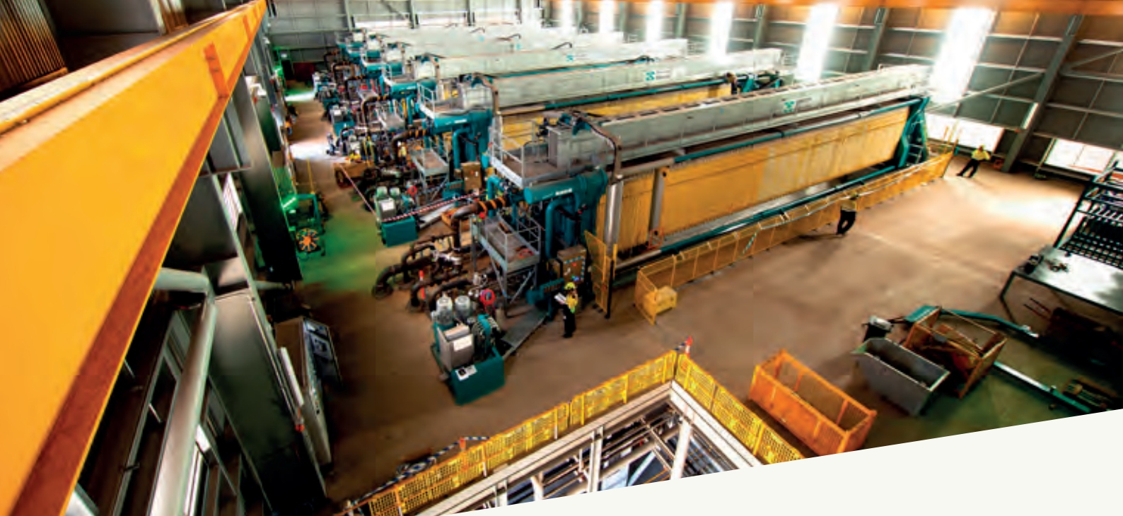
Above: Pinjarra refinery residue press filtration plant prior to commissioning.
