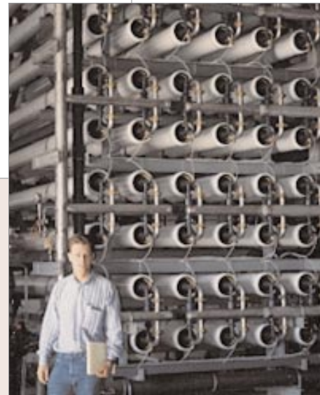
CodeLine pressure vessels serve as the heart of a municipal water filtration facility in Spain.
