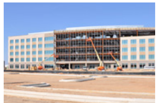
308 Sentinel Drive – under construction in The National Business Park, with direct access to Fort Meade
