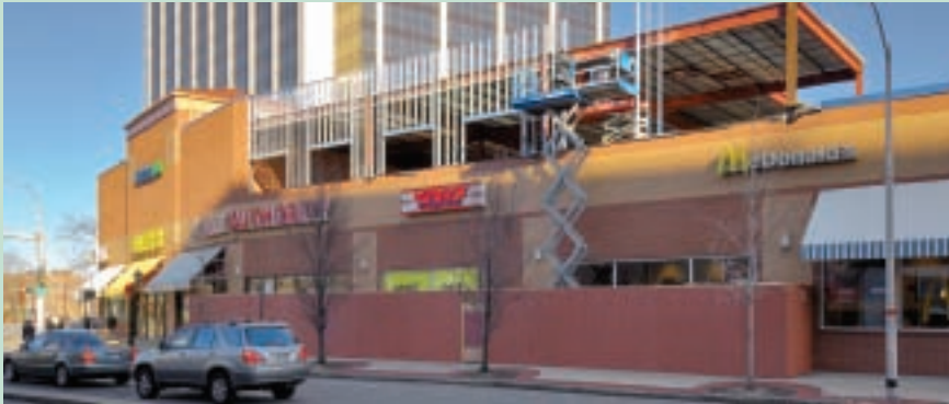
New second floor addition, under construction at Westchester Pavilion in White Plains, New York
