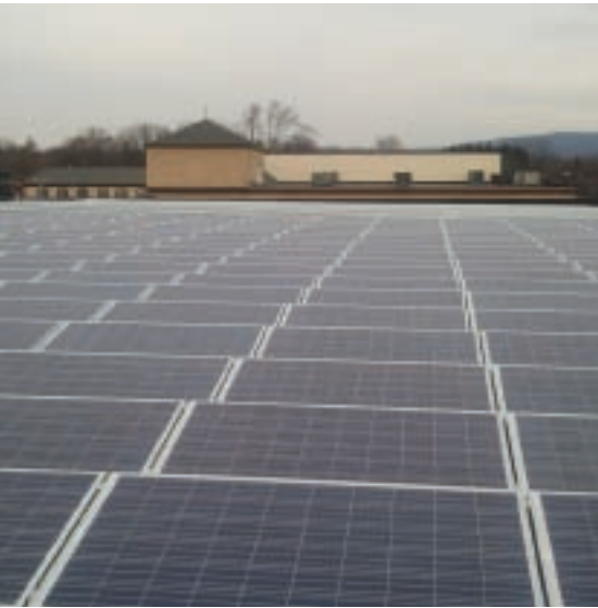
Rooftop solar system at the Valley Ridge Shopping Center, Wayne, New Jersey
