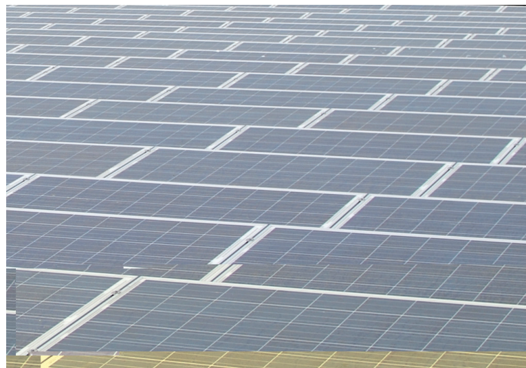
Rooftop solar system at the Emerson Shopping Center , Emerson, New Jersey
