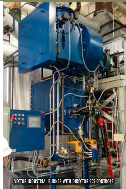
C BURNER WITH NEW AIR DAMPER
