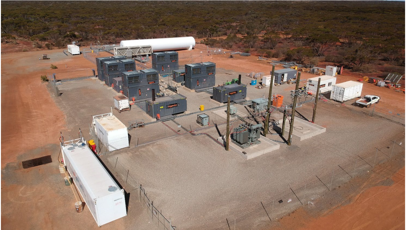
Figure 3: New Power Station with LNG facility in background pre-commissioned
