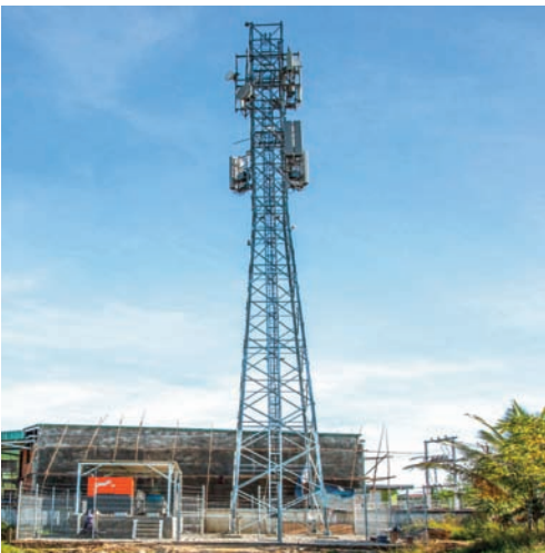
Ground based telecommunications tower
