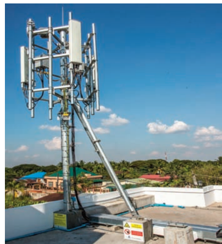
Rooftop telecommunications tower
