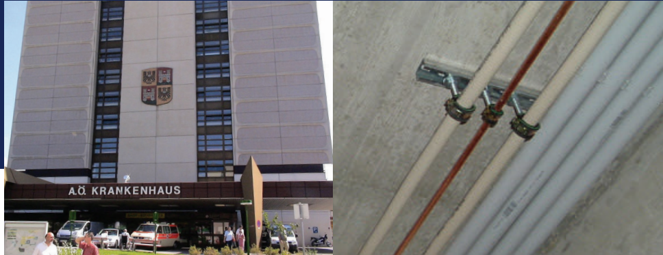
Medical gas piping in Austria.
