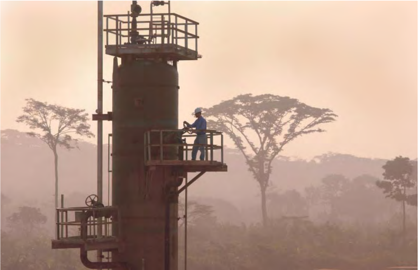
MOVING OIL. Workers finish construction on Pump Station Three at the Belabo site in Cameroon.
