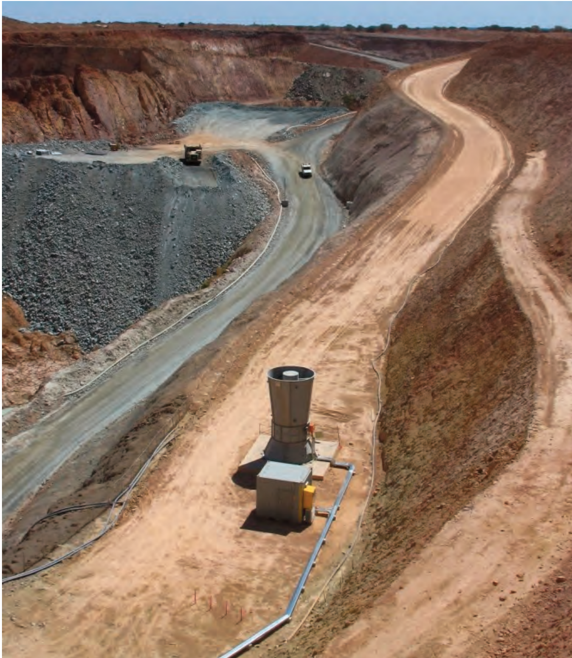
Primary Vent Fan at the Vivien Underground Gold Mine
