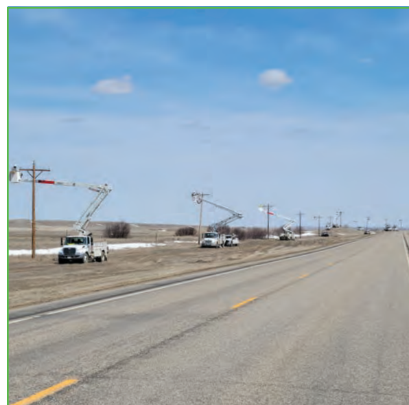
Montana-Dakota Utilities crews work to restore power after unprecedented damage to company facilities from an April blizzard.
