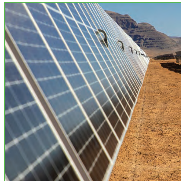
MDU Construction Services Group subsidiary Bombard Renewable Energy finished construction on a 200-megawatt solar facility in Nevada.
