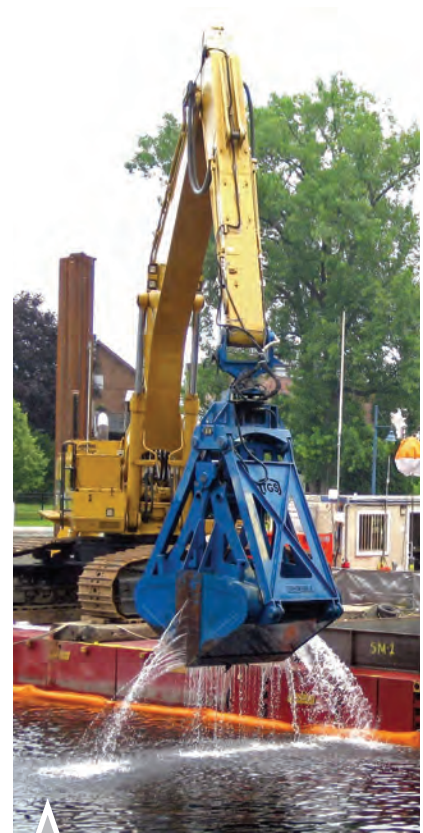
Hudson River PCB Superfund Site Cleanup, New York State. E & E plays a vital role on this nationally recognized, $1 billion environmental restoration project, coordinating stakeholder involvement and developing precedent-setting quality-of-life performance standards with U.S. Army Corps of Engineers, Kansas City District for EPA Region 2.
