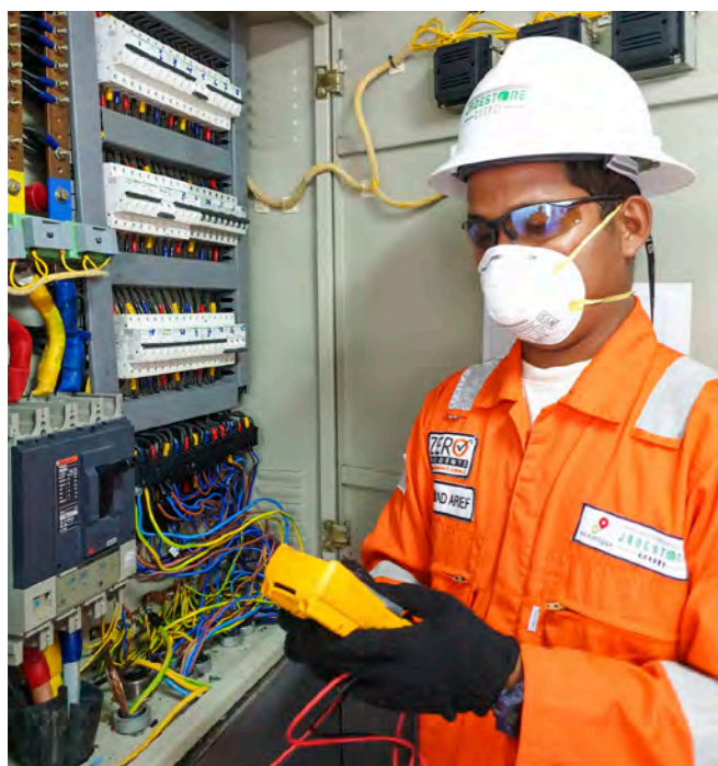
Electrical maintenance and testing at Lemang
