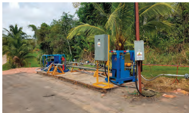
CO2 delivery system at Inniss-Trinity
