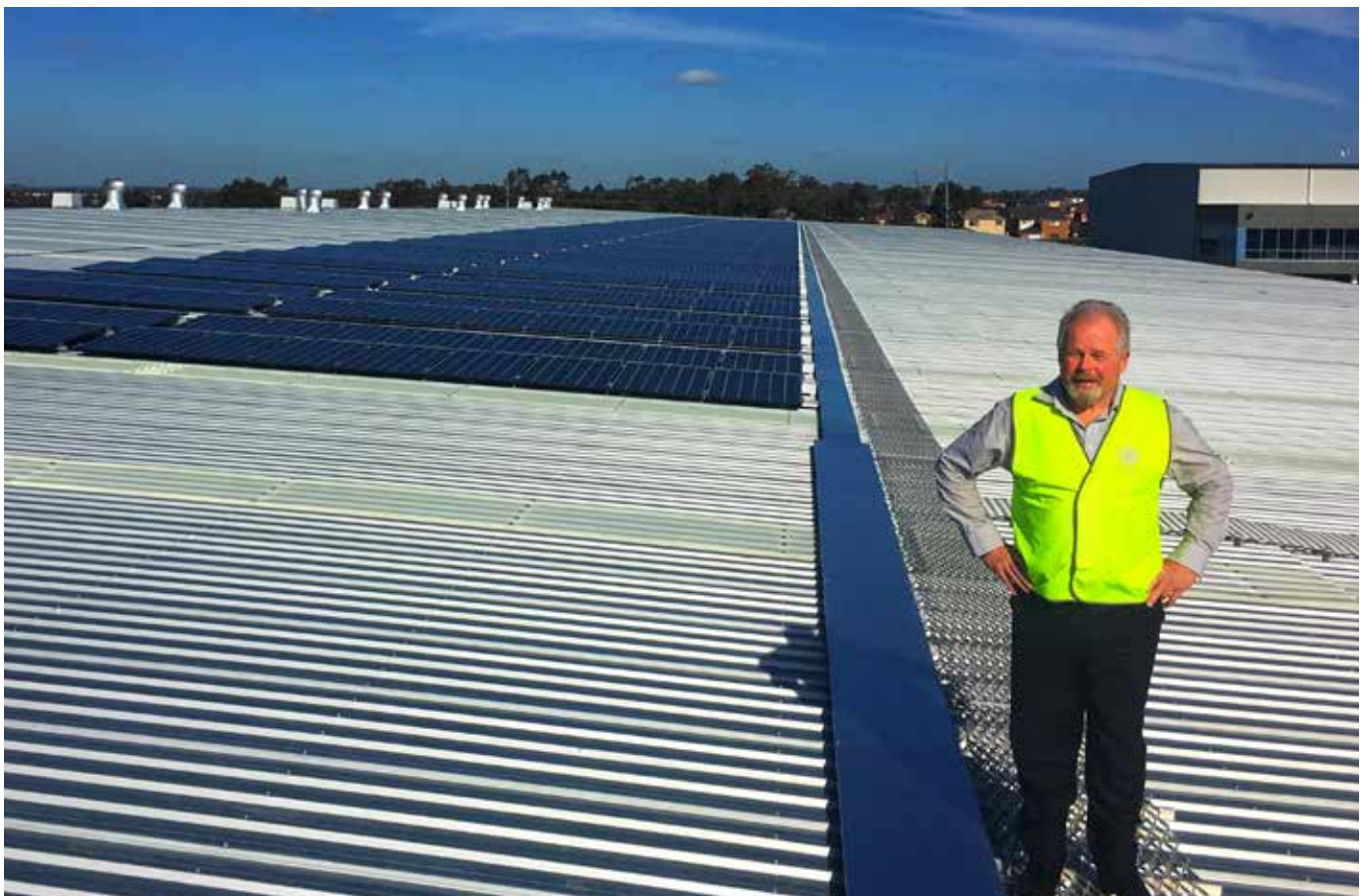
Solar array on the roof at the new Caroma Innovation and Distribution Centre (IDC) at Prestons NSW.
