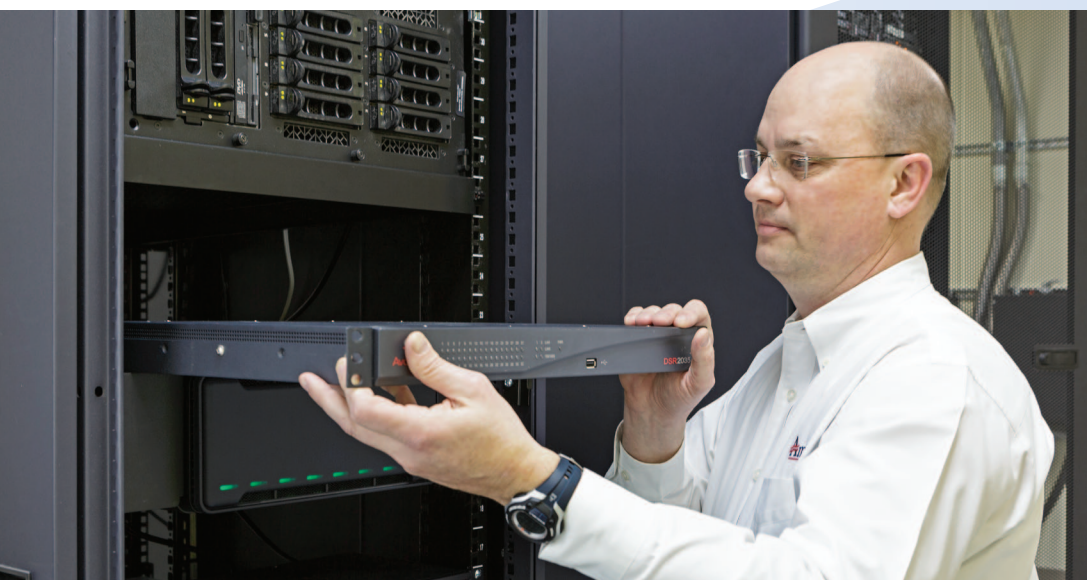
Shan Venable, VP and System Architect Manager for our Information Technology Division, is installing a server management appliance in one of our data centers.
