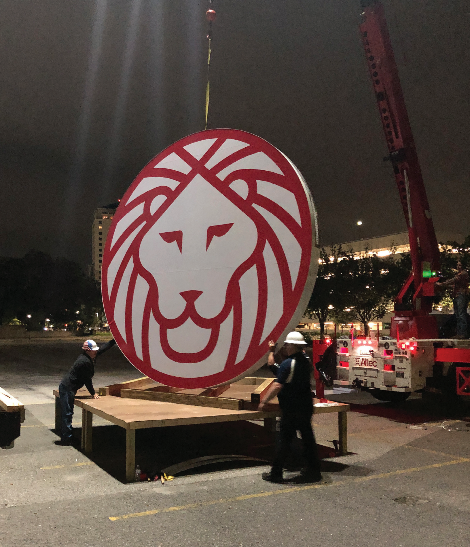
Ameris Bank's new brand deployed in November 2019, with signage crews starting to install the new logo on facilities across our footprint. In Jacksonville, Florida, signage crews prepared for the installation by helicopter of the new Ameris Bank logo atop the 27-story Riverplace Tower.
