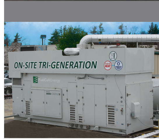
Tri-generation fuel cell power plant supplying ultra-clean power, heat and hydrogen to the FuelCell Energy manufacturing facility in Torrington, Connecticut, USA
