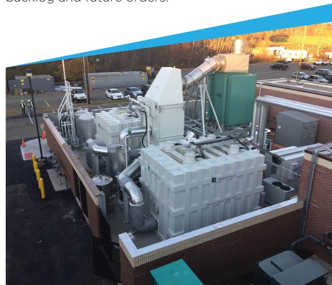
2.2 megawatt fuel cell plant generating continuous power and usable heat. The fuel cell is the sole power source for a state-of-the-art town microgrid providing power to critical facilities including: the local high school, town hall, library, firehouse, police station, public works facility and senior center.
