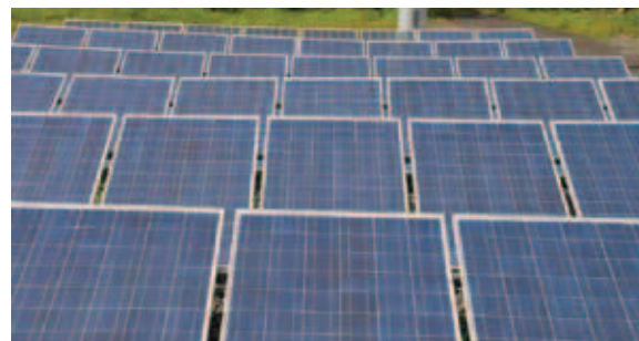
Solar Photovoltaic system installed at RCP
