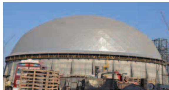
Coke dome with Stacker and Re-claimer
