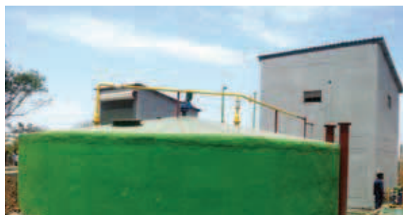
Biogas plant installed at RCP
