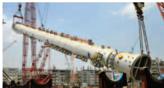
1.4 MMTPA refinery off-gas cracker to be among the world's largest ethylene crackers
