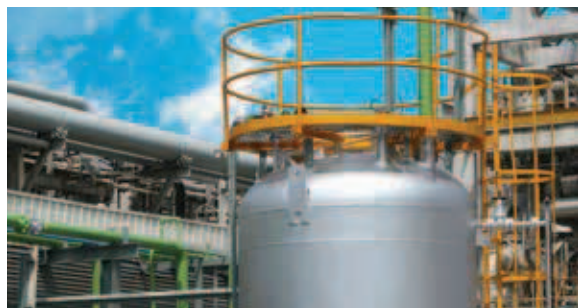
Gas dehydration units at Gadimoga onshore terminal
