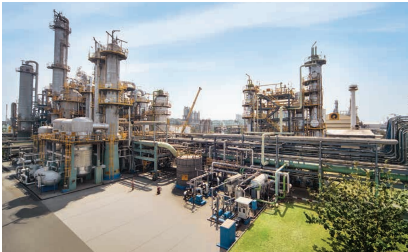
Petrochemical Plant at Hazira manufacturing division
