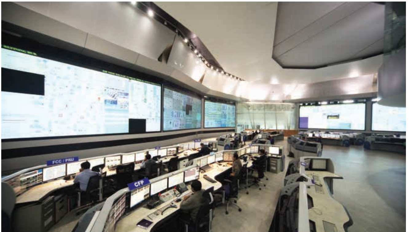
Jamnagar SEZ control room
